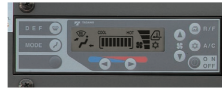
Air conditioner Hot-water heater and air conditioning.
